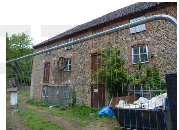
Hempstead Mill, which is vacant though there appears to be building work on the site. The building also has modern uPVC and timber windows that are out of character with the historic building and Conservation Area
